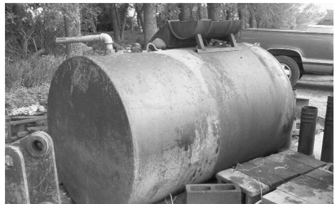
Even waste oil tanks have to be considered if they exceed the minimum size and volume requirements of the SPCC regs.
